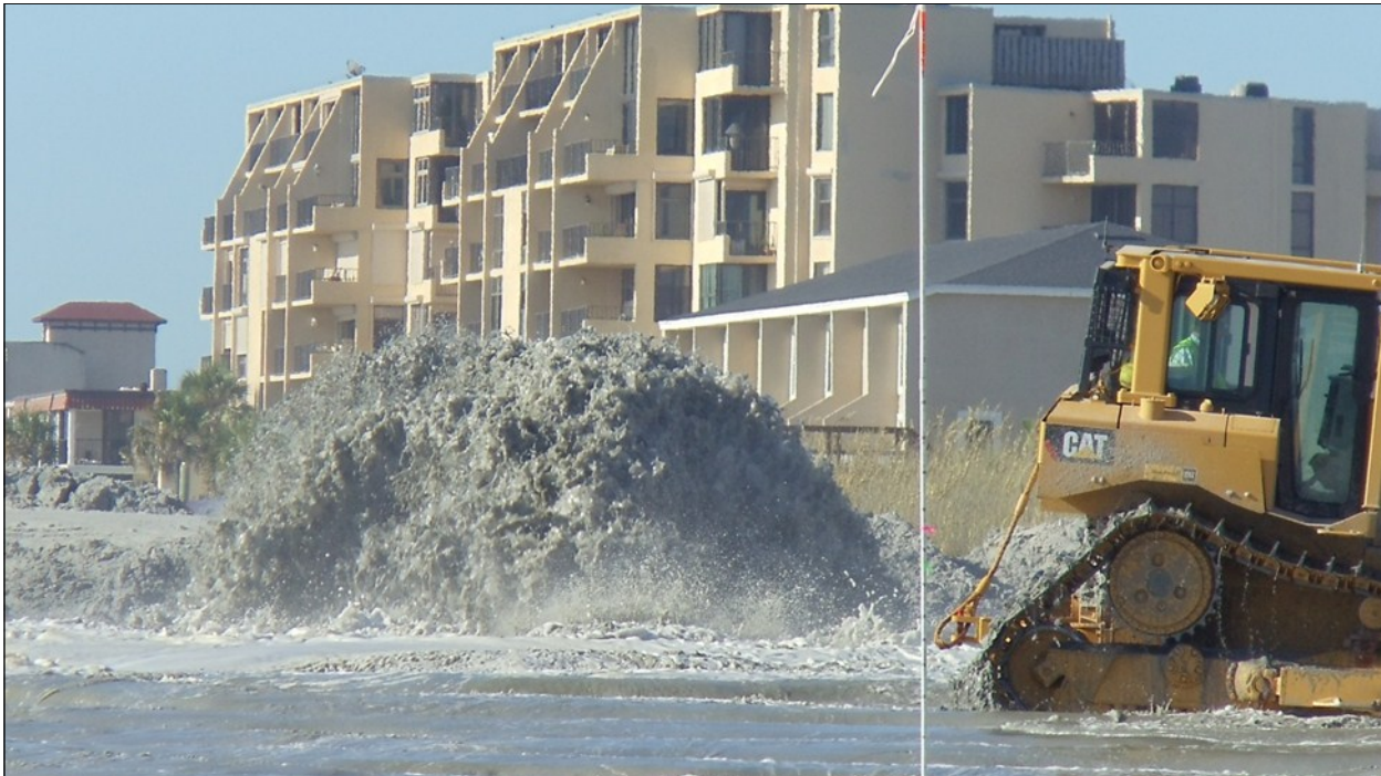
Progress has been swift on the Duval County hurricane and storm damage reduction project. Here, sand is being pumped on the beach in front of the city of Jacksonville Beach. Two dredges are working simultaneously on the project. (Photo by Jim Vecchito)
