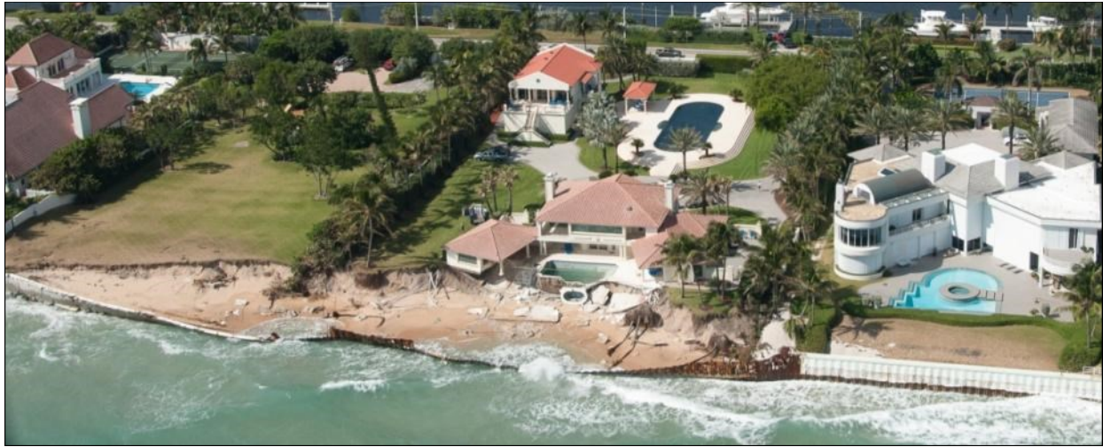
Undermined (and overtopped) Seawall in Manalapan
