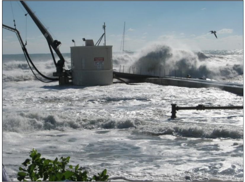
The Lake Worth Inlet Sand Transfer Plant during Hurricane Sandy
