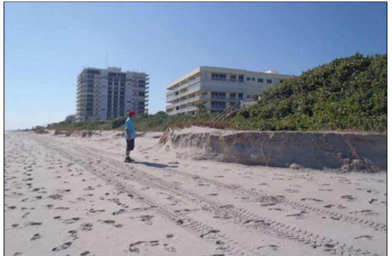
Cutline: Brevard County South Reach: Scarping of protective dune – evident that entire berm was recently submerged.
