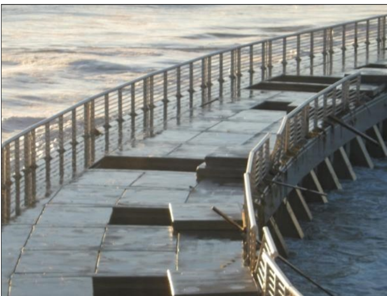
Damage to the north jetty at the South Lake Worth Inlet
