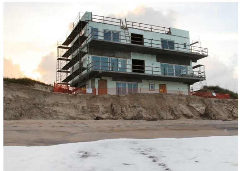
This House under construction directly on the dune at Vilano Beach clearly illustrates the need for dune protection setback.
