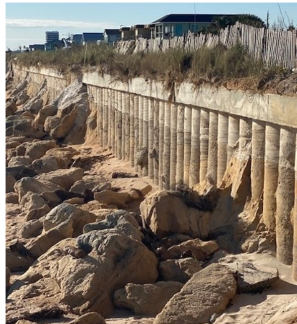
Figure 4: Scour from Hurricane Ian exposed up previously buried rubble boulder near the toe of the wall (source: Lead author's photo).
