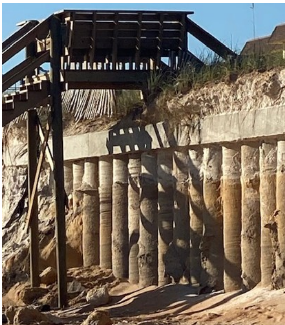
Figure 3: Scour from Hurricane Ian exposed up to 13-feet at the face of buried secant-pile bulkhead/seawall (source: Lead author's photo).
