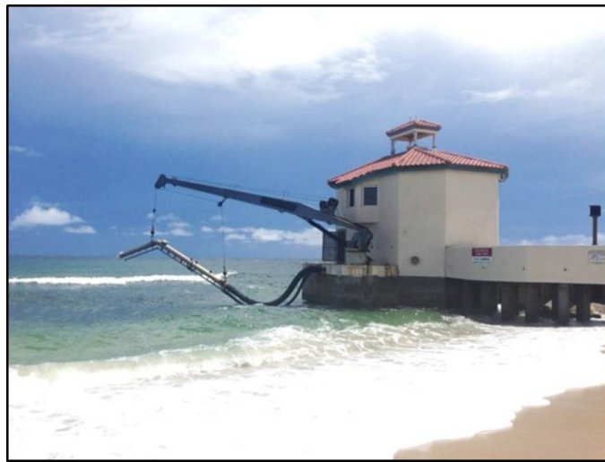
Figure 3. Sand Transfer Plant at South Lake Worth Inlet (Photo: Pierro, Sept. 2015).
