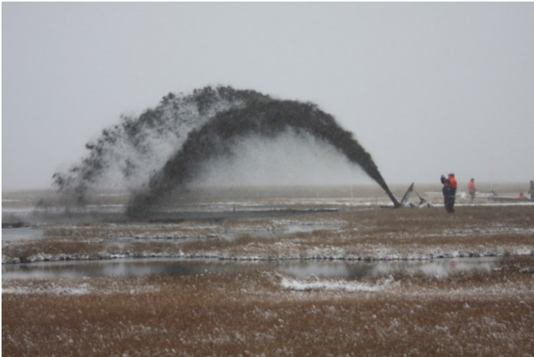
Figure 2: Thin-layer placement during the New Jersey Avalon Pilot Project (Chasten and Goldberg, 2016).
