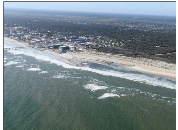
St. Augustine Shore Protection Project at early stages of construction near R141 in February 2018 photo by W.G. Weeks.
