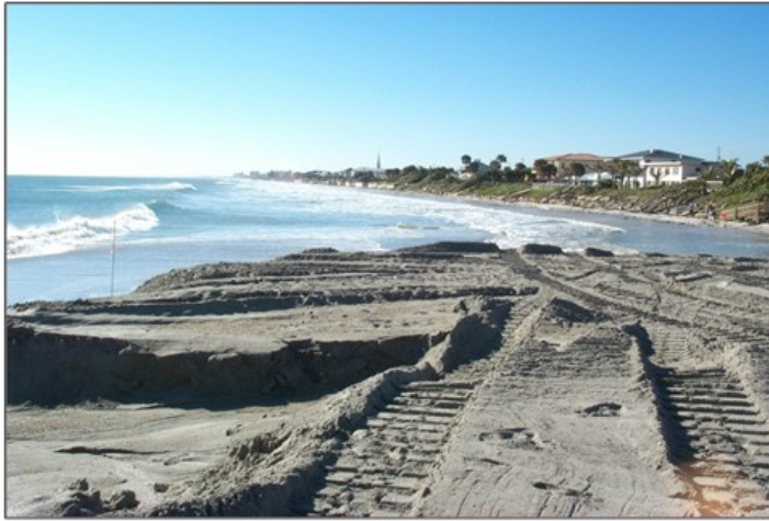
Shoreline in the Brevard County North Reach in 2000 (start of initial construction)
