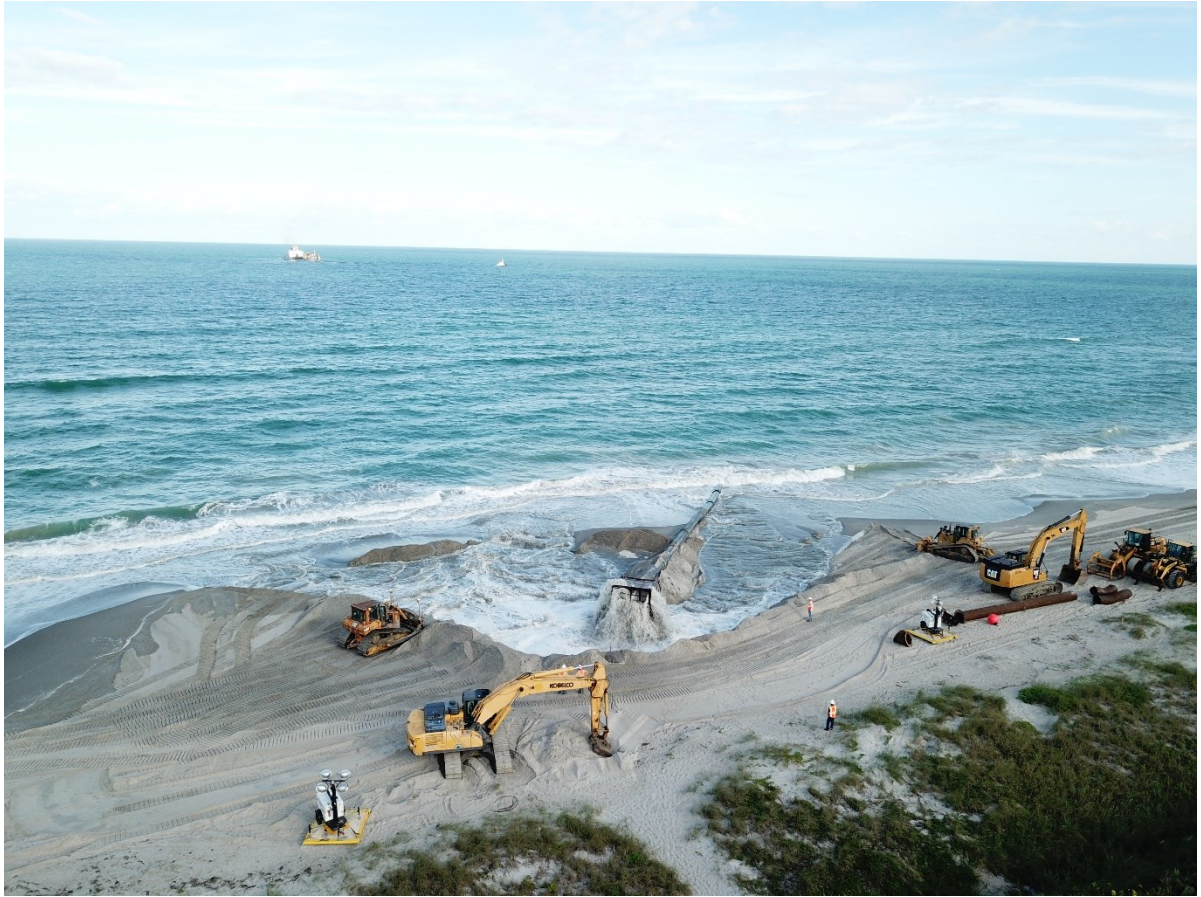
Construction of the Brevard County, FL Shore Protection Project by The Dutra Group during the 2019 - 2021 renourishment Credit: U.S. Army Corps of Engineers
