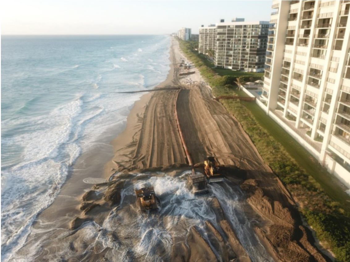
Construction of the St. Lucie, FL Coastal Storm Risk Management (CSRM) project was completed by Great Lakes Dredge & Dock in May, 2022. Credit: U.S. Army Corps of Engineers
