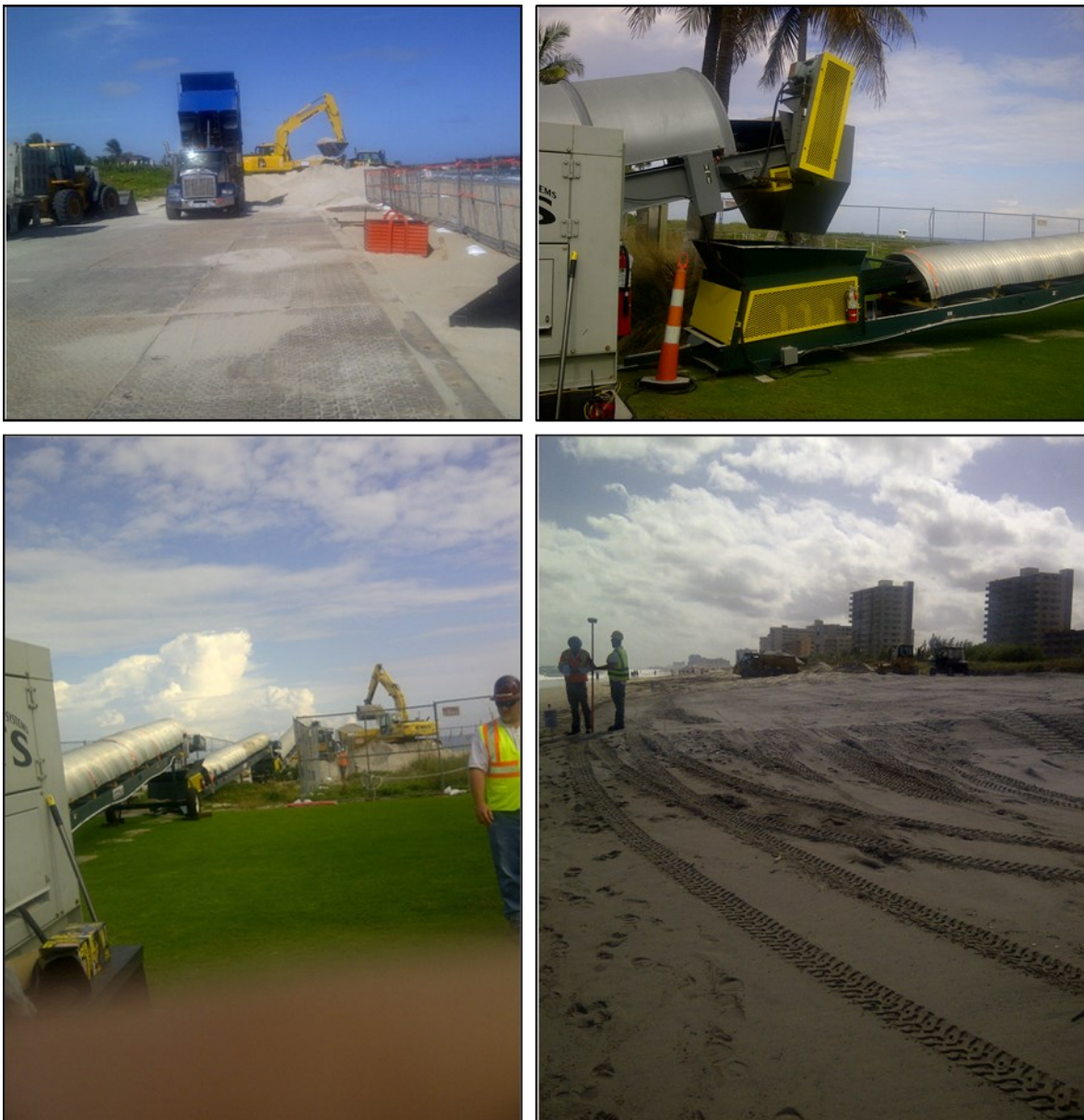
Figure 2: Photos of the ongoing construction of the Broward County Beach Erosion Control Project.
