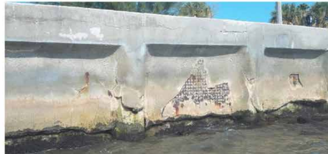
Figure 3-6 Loss of Shotcrete Exposing Mesh
